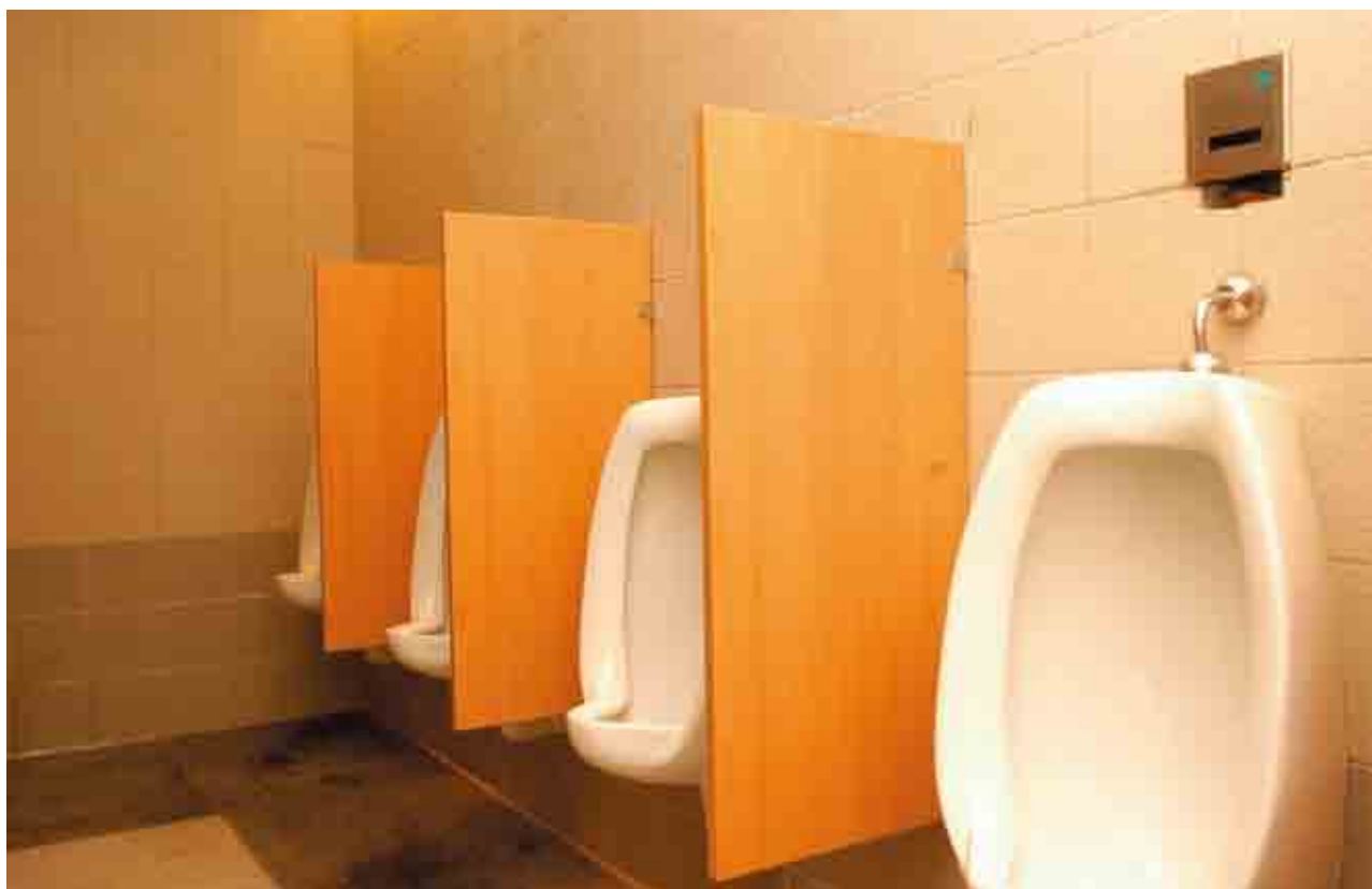
Toilet partition boards 浴廁隔間板
